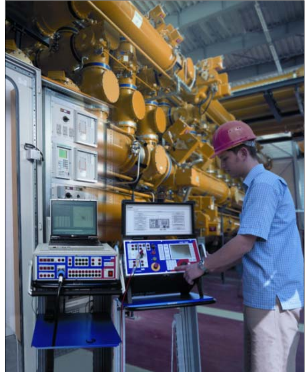
Fig. 13: Secondary test set CMC 256 and primary test set CPC 100 from OMICRON in use
